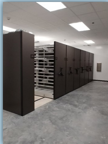
Mobile Storage System
